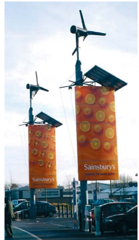
Wind energy turbines
